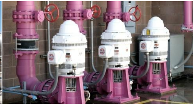
Automated Asset Management
